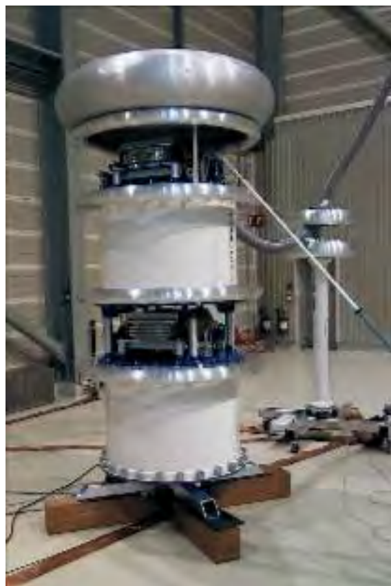
Test transformer cascade rated 200 kV; 0.7 A
